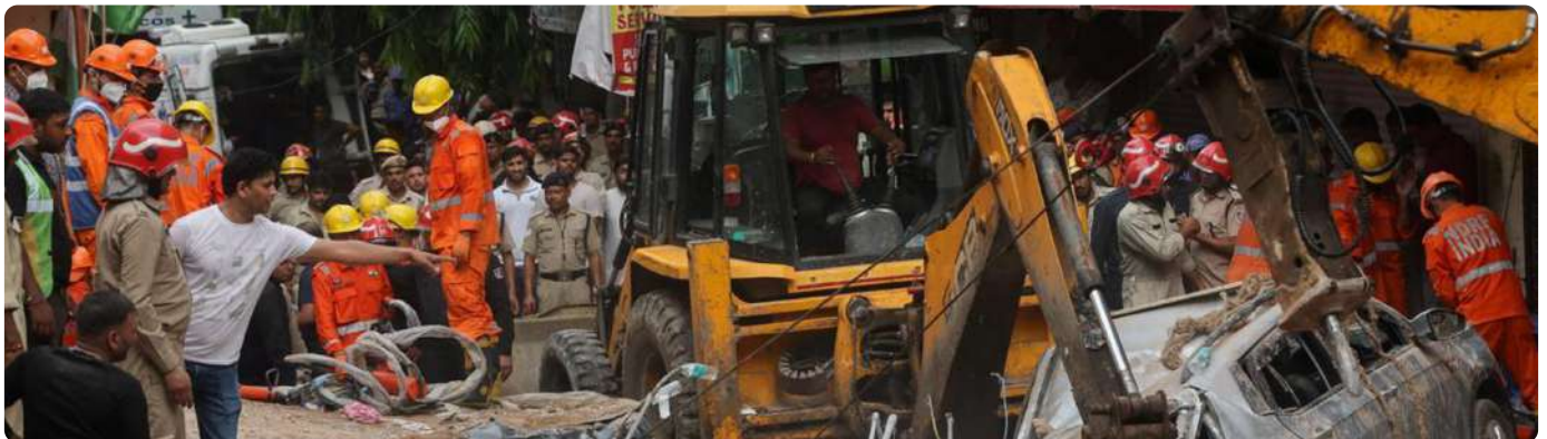
NDRF and rescue teams clear debris at the collapse site in Satya Niketan.
