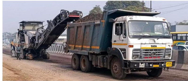
In the works: Reconstruction of a road begins near NH-709B, Sisana village, in Baghat, Uttar Pradesh on February 4. ANI
